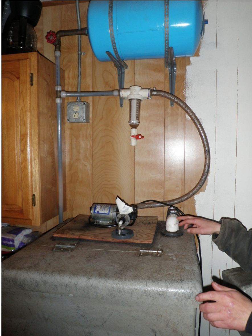
Water holding tank and pump system typical of rural Alaskan homes. Photo courtesy of B. Lefferts.
